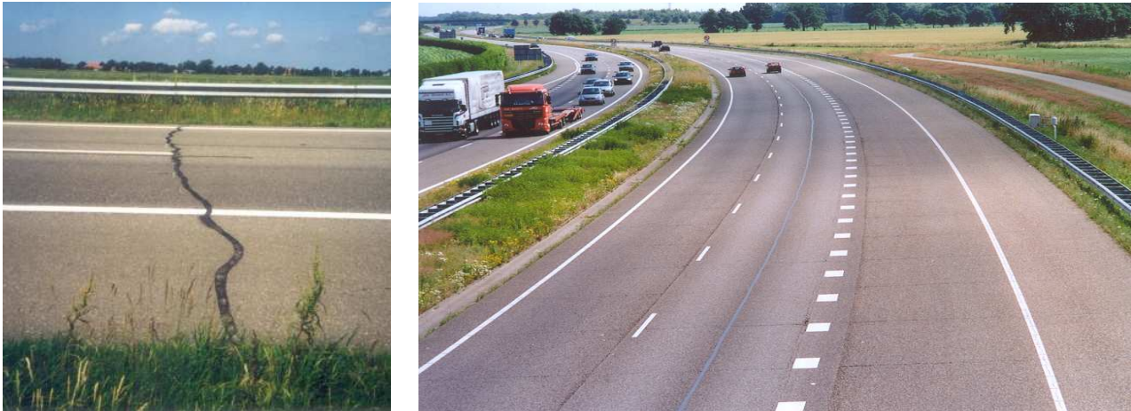
Figure 2. Typical reflective cracking on a cement treated base (left) and concrete slabs (right)
