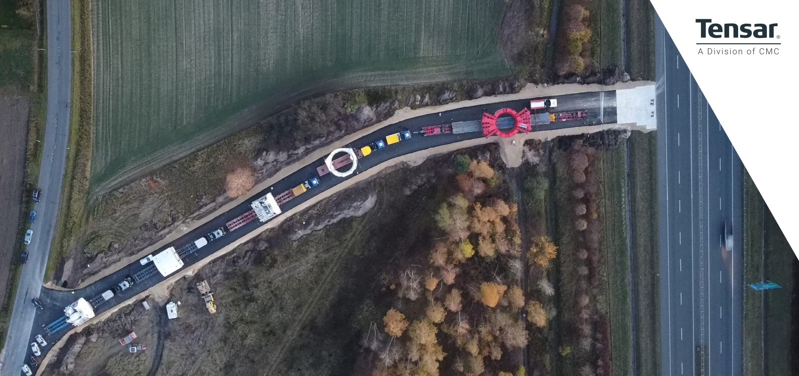
The 214m long link road was designed for the 14 specialist transporters carrying components of the 4,000 tonne tunnel boring ma-
