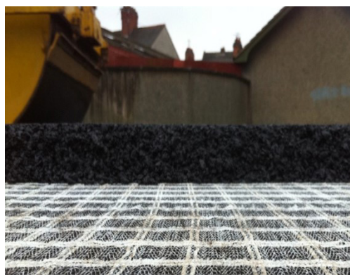
Tensor Glasstex P100 is laid to mitigate against reflective cracking and limit its spread into the newly laid asphalt course
